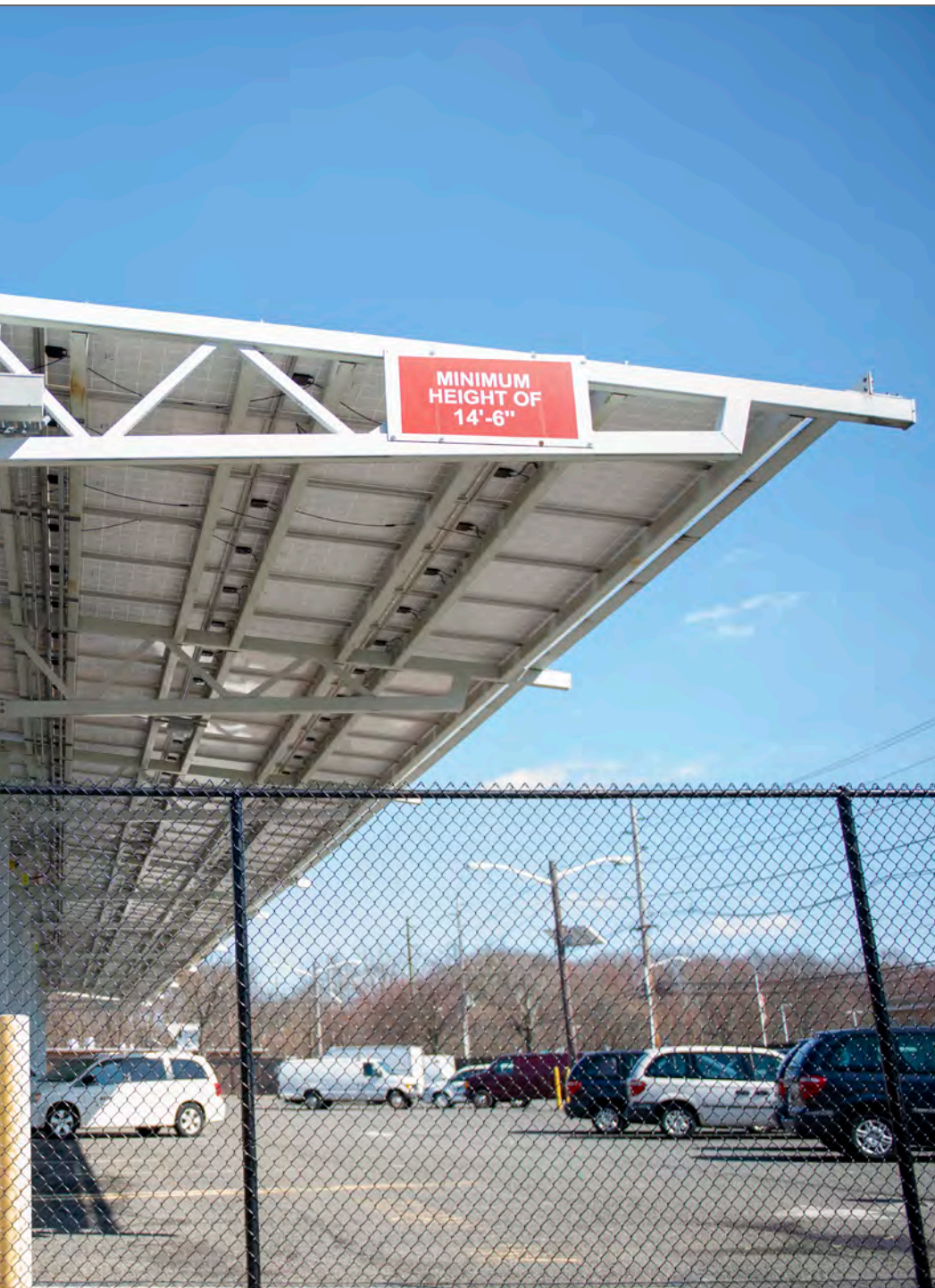
Solar Canopy. Source: Donna Brennan, Bergen County
