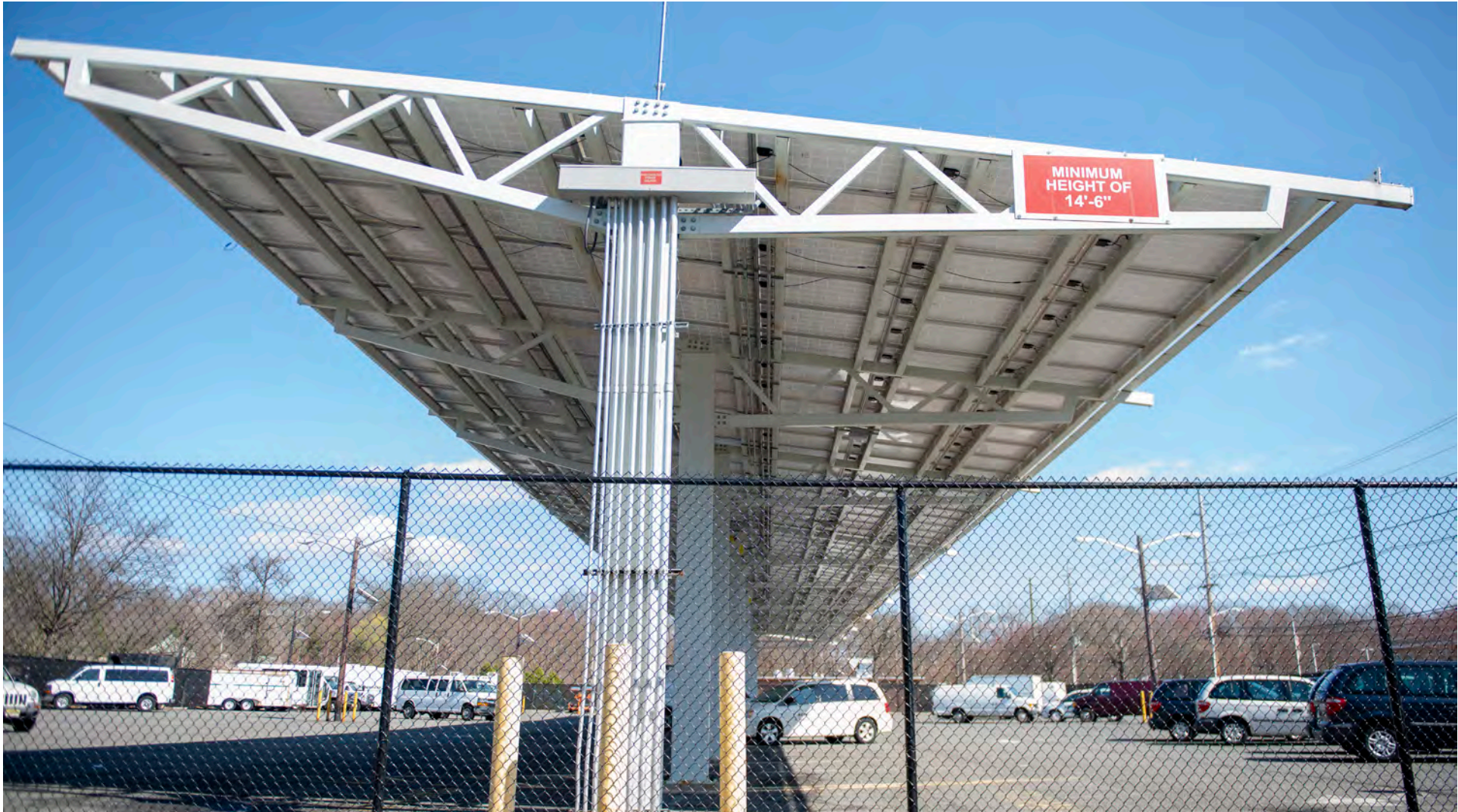
Solar Panels. Source: Donna Brennan, Bergen County
