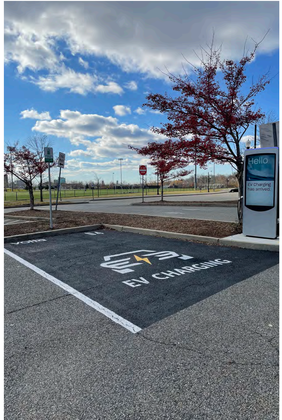
Electric Vehicle Charging Station at Overpeck County Park. Source: Colliers Engineering & Design
