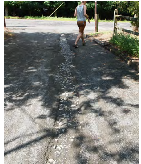
Erosion on driveway (Image 3.6.5.5)
