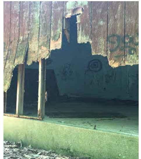
Run down building (Image 3.2.8.2)
