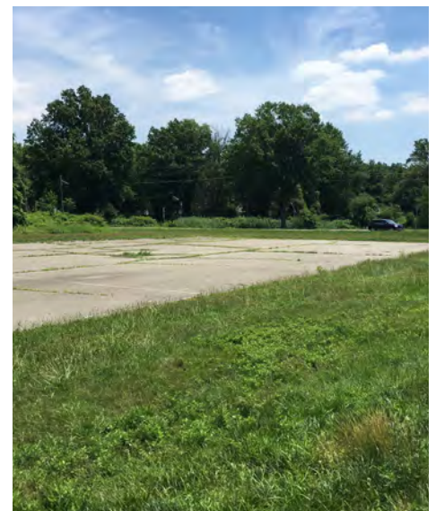
Abandoned concrete slab (Image 3.1.2.5.5)
