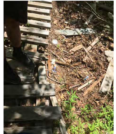
A half-broken wooden bridge (Image 3.3.3.3)
