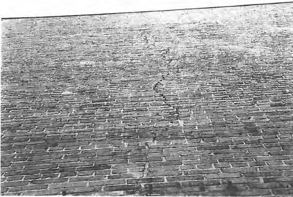
Photo 54 Close up of typical vertical crack. See attached drawings for vertical crack locations. Cracking should be repaired.
