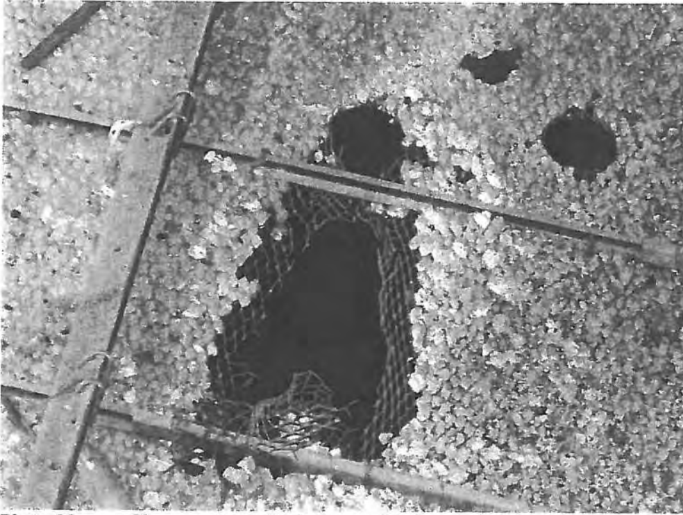
Photo 33 Closeup view of hole in metal lath and plaster ceiling.
