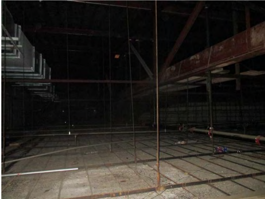
Photo 3 General view of suspended ceiling support system
