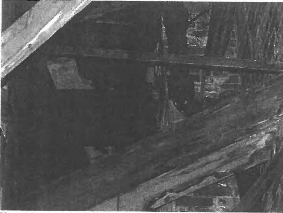
Photo 27 Water infiltration and efflorescence on the exterior walls and wood framing at roof.
