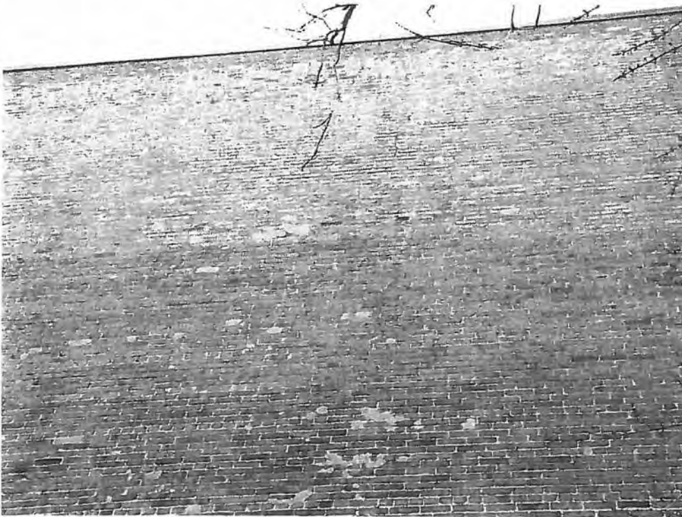
Photo 52 Close up of wall with cracks, missing bricks or loose bricks. The conditions should be repaired.
