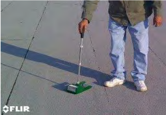
PHOTO 1 Lower Roof Section: Tramex meter was place on roof surface every 2-4 feet in grid pattern.
