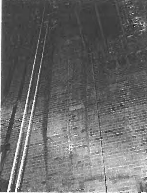
Photo 41 Vertical crack in pilaster proscenium wall stage right. Condition must be mitigated.
