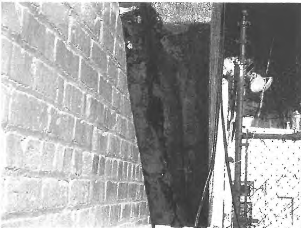
Photo 58 North east thrust block does not extend below grade. Steel plate is corroded and concrete is cracking. The condition should be repaired.
