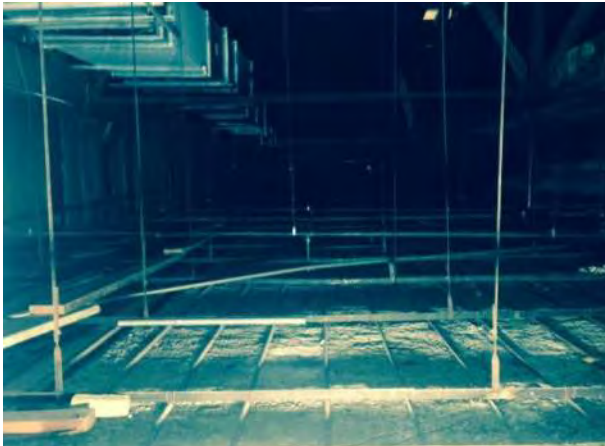
Fig. 1 Typical view across the plenum indicates a systematic and orderly layout. Attached to the plaster by wires, the typical Chicago Bar system is spaced at 16: with the opposing angle irons at 5' centers. Verticals bolted to these are 1" X 1/8" straps.
