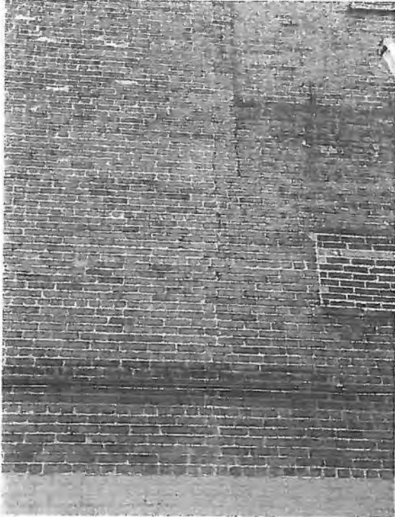
Photo 49 Vertical cracking in brick masonry. Condition should be mitigated.
