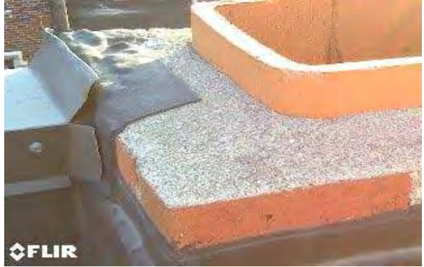
PHOTO 8 Lower Roof Section: Metal cap over chimney wash is recommended be installed and lapped over metal coping cap.
