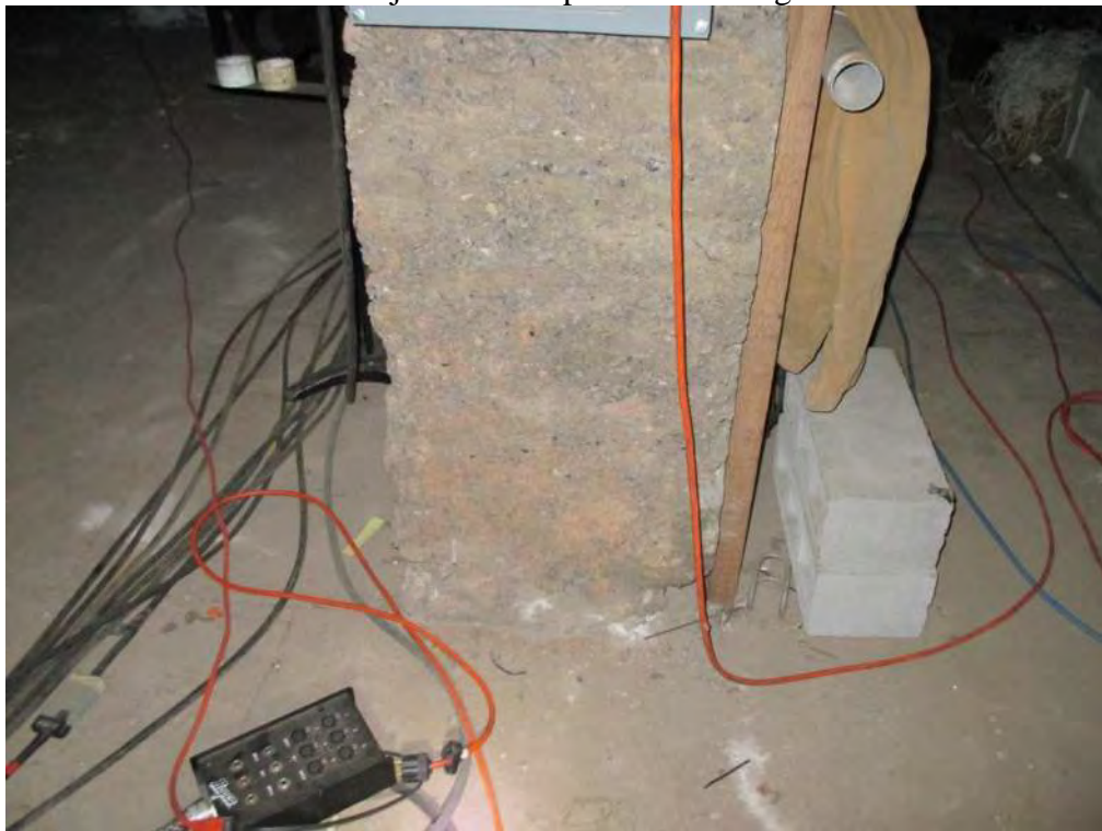
Photo 18 Honeycombed concrete column under proscenium stage
