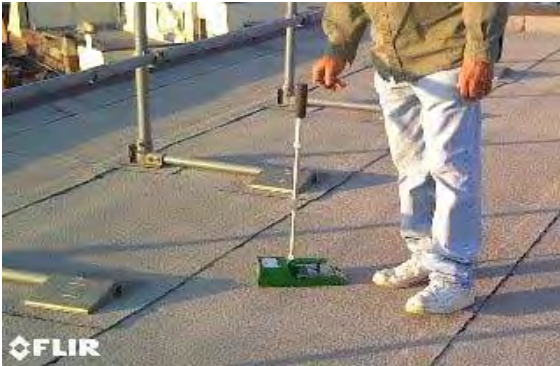
PHOTO 9 Upper Roof Section: Tramex meter was place on roof surface every 2-4 feet in grid pattern.
