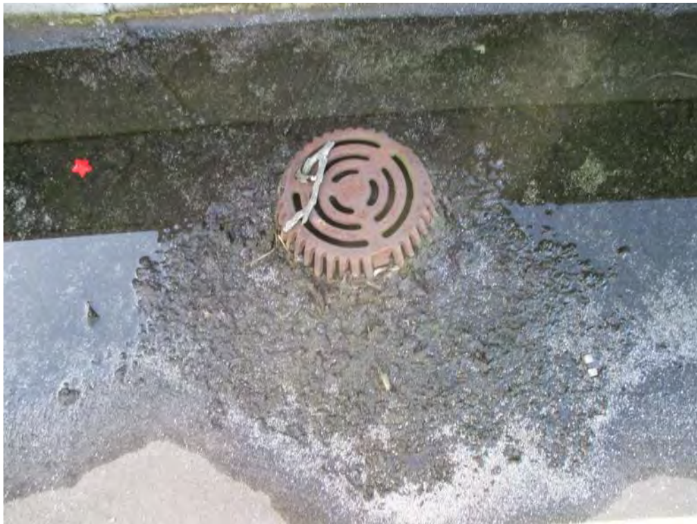
Photo 6 Clogged roof drain
