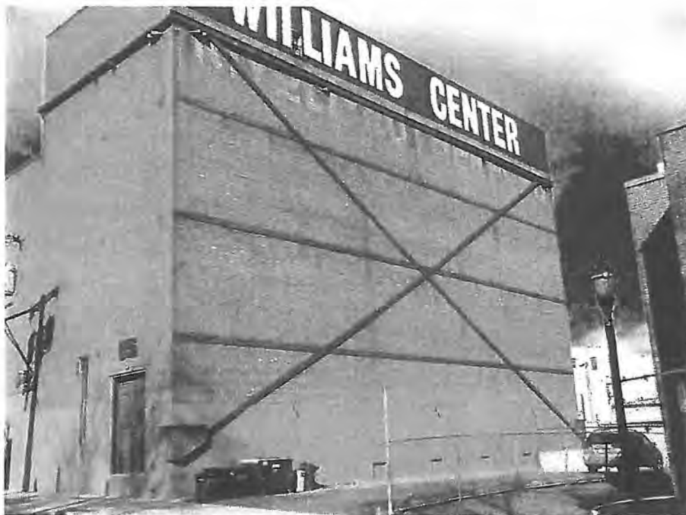
Photo 1 East Elevation (viewed from Spring Dell). Note the steel strap bracing on the wall at the rear of the stage. There exist the steel channel belts at the top of the stage bulkhead.
