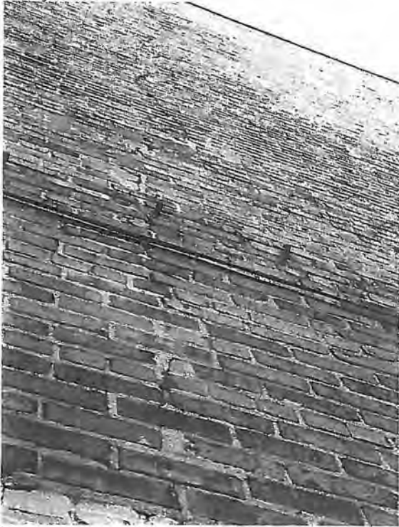
Photo 53 Close up of brick masonry with loose mortar. Conditions should be repaired.
