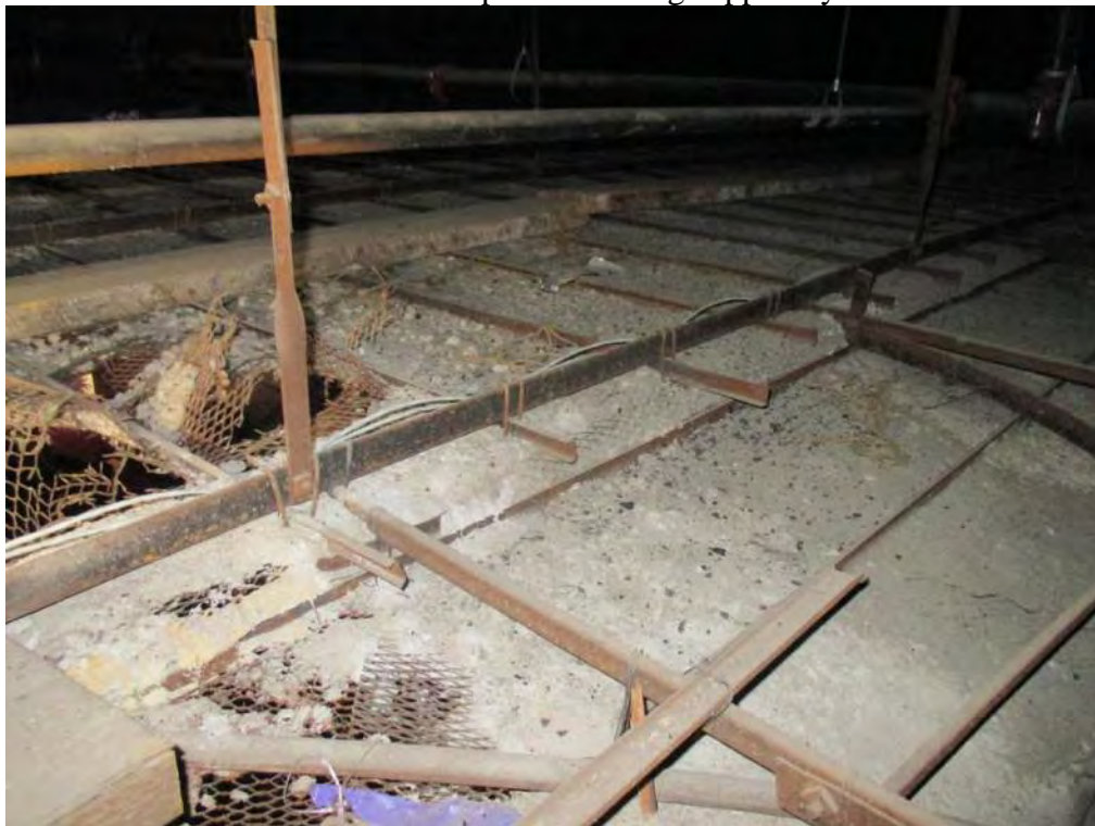
Photo 4 Damaged area of suspended ceiling.
